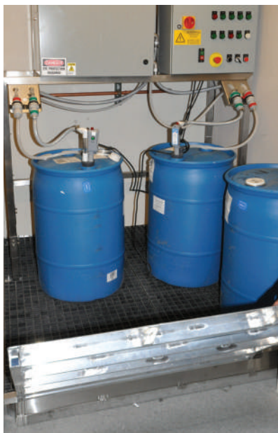
Containment platform with drain pan and leak sensor
